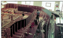
A temporary outer ring of the Biscuits slide layers. The temporary single splines in the lower center and the plate will come used to join the locations of the track. The cone were installed, then the final spline substructure was finished.
