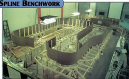
The hub-and-spoke web is ready for the Biscuits. (Biscuits slide layers during the early stages of construction. Note the blue spline scaffold and conventional 1/2-inch-thickness scaffold and track in place on the right.)
